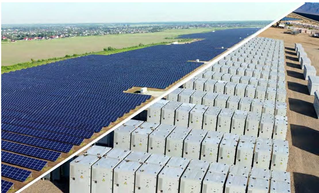
Figure 6. Onsite generation and storage is needed at a large-scale to provide the scale of backup power required for data centers.
