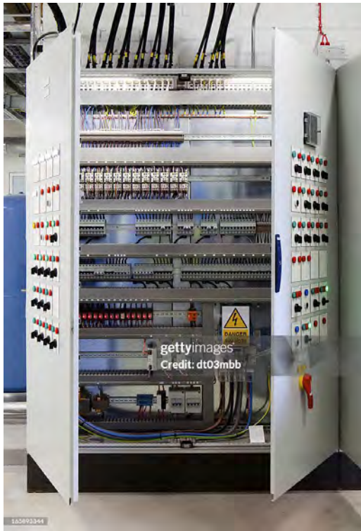
Image Source: https://www.gettyimages.com/detail/photo/systems-control-cabinet-royalty-free-image/165893344
