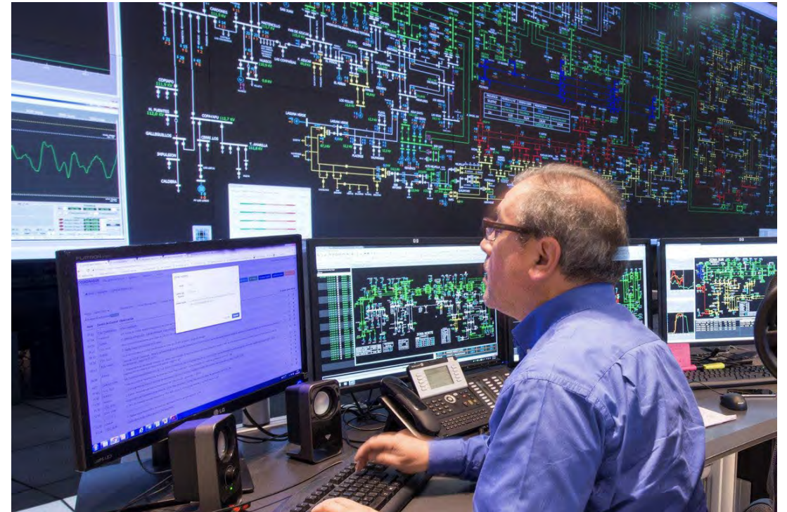
Image Source: https://www.saskwind.ca/power-and-renewables/system-operators/
